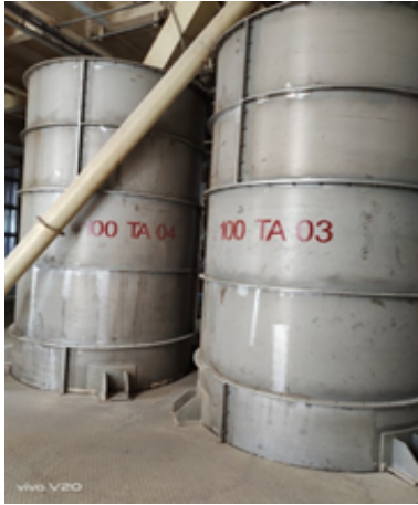
Intermediate Storage Tank
