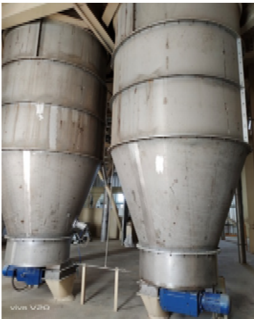
Intermediate Storage Tank
