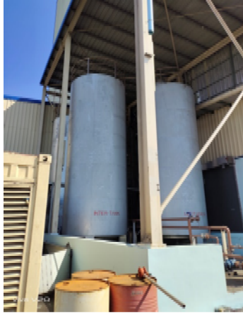
Oil Storage Tank
