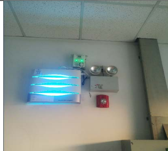
Emergency Light & Sign
