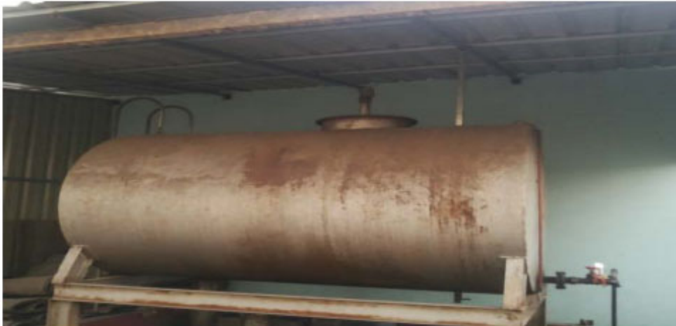
Fuel Storage Tank for Generator
